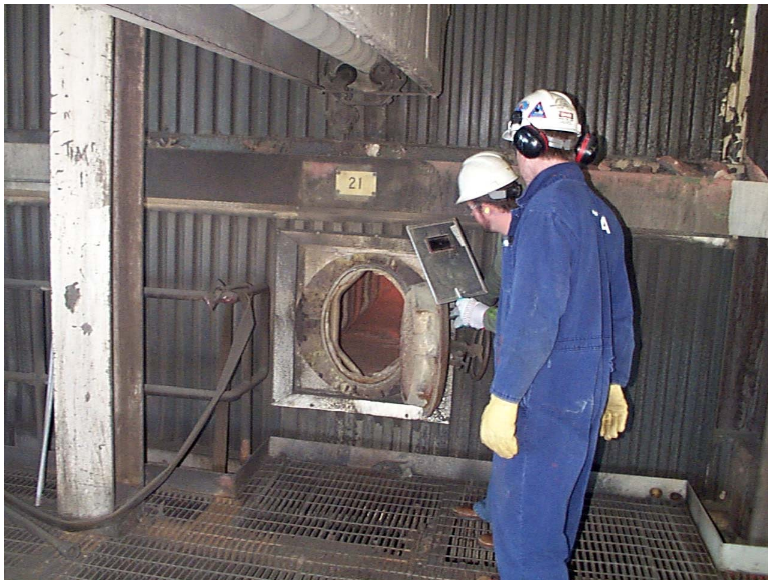
Typical access point to Site 1 boiler
